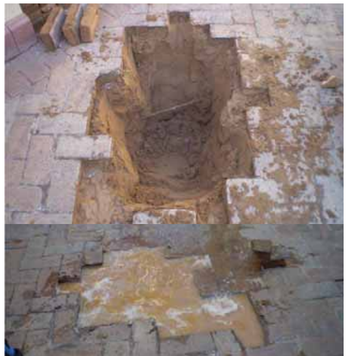
Found the leak
