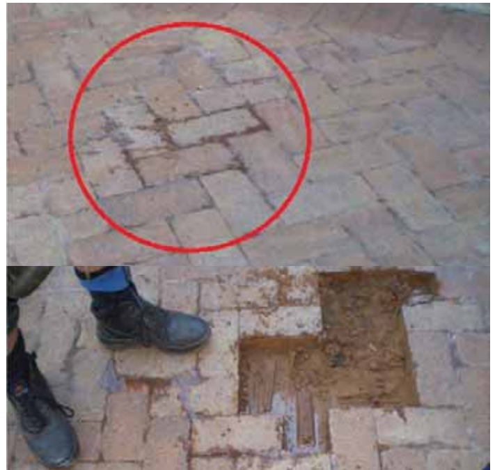
Finding the leak
